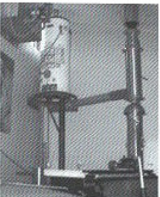
Fig. 8 Pablo Soto's secondary air-to-liquid heat exchanger reclaims heat after his recuperator to heat the adjacent studio space via a radiant floor
